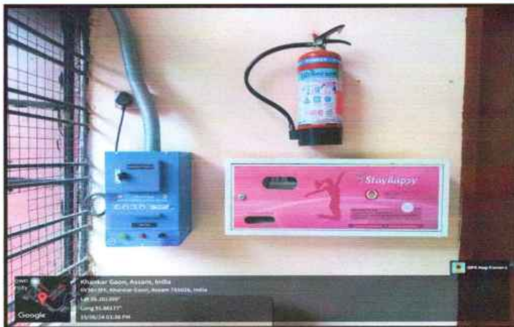
Fig.3 (b):- Sanitary Napkin Incinerator: Girl's Common Room
